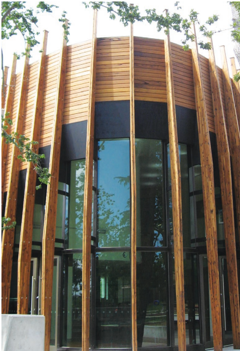
■ Camberwell Girls Grammar School ... two coats of Cutek on DuraBeam silvertop ash.
